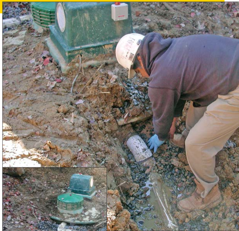
Above, Juan Gonzalas clears soil from around the pipe to check the connection to the Aqua Safe treatment unit. At left, the septic tank riser appears in the foreground; then the riser on the Aqua Safe pretreatment unit and its control, housing the air compressor and electrical components. (Photos courtesy of Superior Plumbing)
